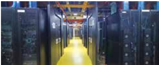
Precise cooling at our data centre to drive energy efficiencies
